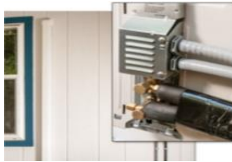
Line set properly insulated
