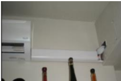
Indoor units located below window and too close to ceiling
