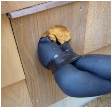
Envelope penetration not sealed properly
